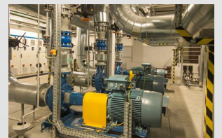
Data Center Pump Skid
