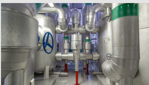
Cooling Piping Systems
