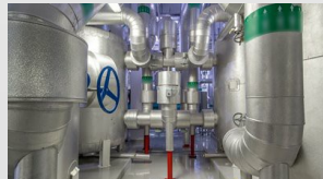
Cooling Piping Systems
