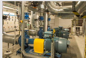
Data Center Pump Skid
