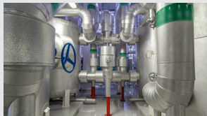
Cooling Piping Systems
