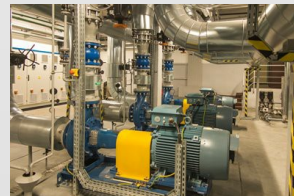
Data Center Pump Skid
