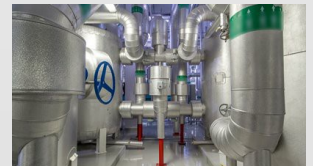
Cooling Piping Systems
